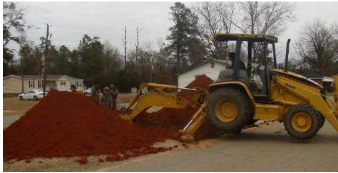
Even seemingly simple repairs can be costly if happening at the wrong time or place. The City of Jeffersonville would spend nearly $50,000 to repair this broken water main under U.S. 80.
